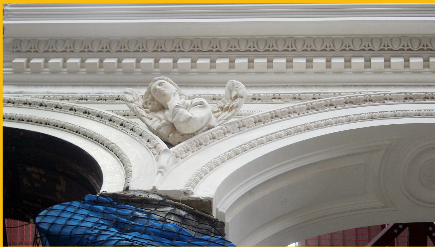
Some of the new trial plasterwork undertaken at the archways above the pillars.
